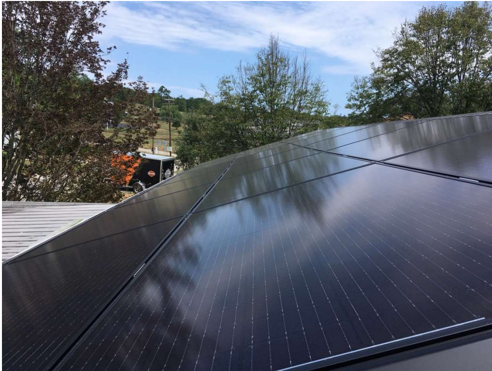
Figure 20 – Solar arrays on both roofs have greatly diminished our grid usage
